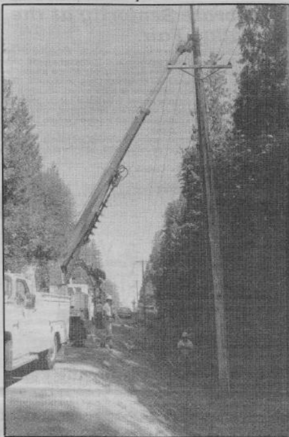
Going UP! Peninsula Light Company crew installs a new "tall" pole along Lackey Road in the central Key Peninsula area. Staff photo by Hugh McMillan
